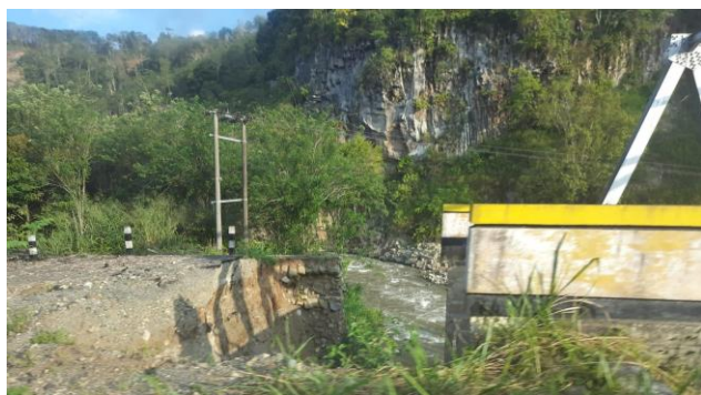
Figure 1. Collapsed soil under the road
