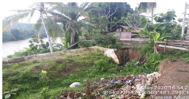
Figure 2. Collapsed soil in the retaining wall
